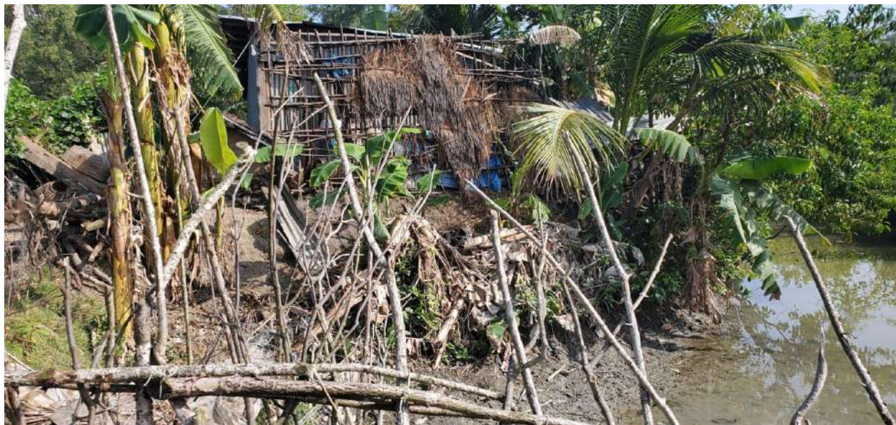
Photo: Cyclone affected house of Md. Parvez Shunnerchor (3 No ward) Hatiya Upazila
